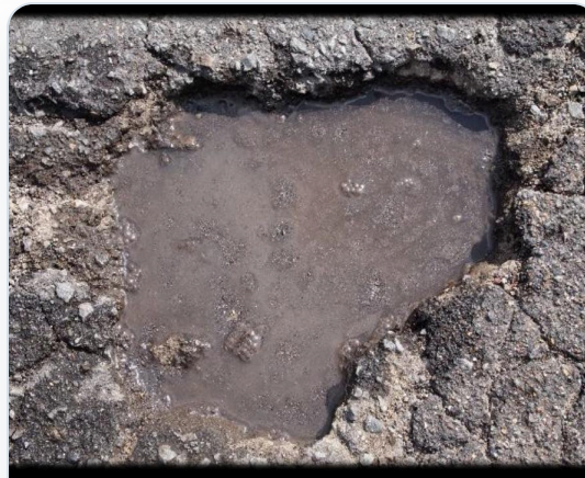
Wet and broken pavement area
