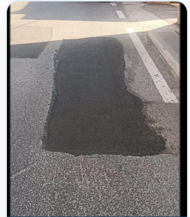
Stable surface after use
