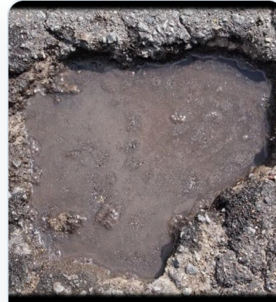
Broken pavement area repair
