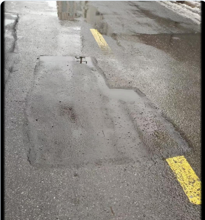
Road condition after snow
