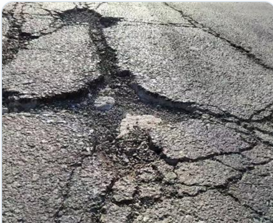
Typical pothole and crack damage
